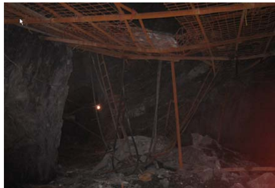
图 13 105 # 矿体内 1 # , 2 # 采空区间重叠顶板冒落情形 Fig.13 Caving state of overlapping roof between goafs #1 and #2 in orebody #105
